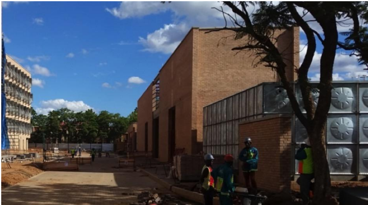
The bulk services for Erf 2503 have been centralised into a service building supporting all the 2016 and 2017 buildings.
